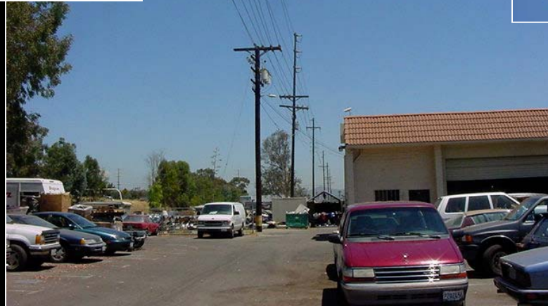
Distribution Pole for Monitoring Equipment
