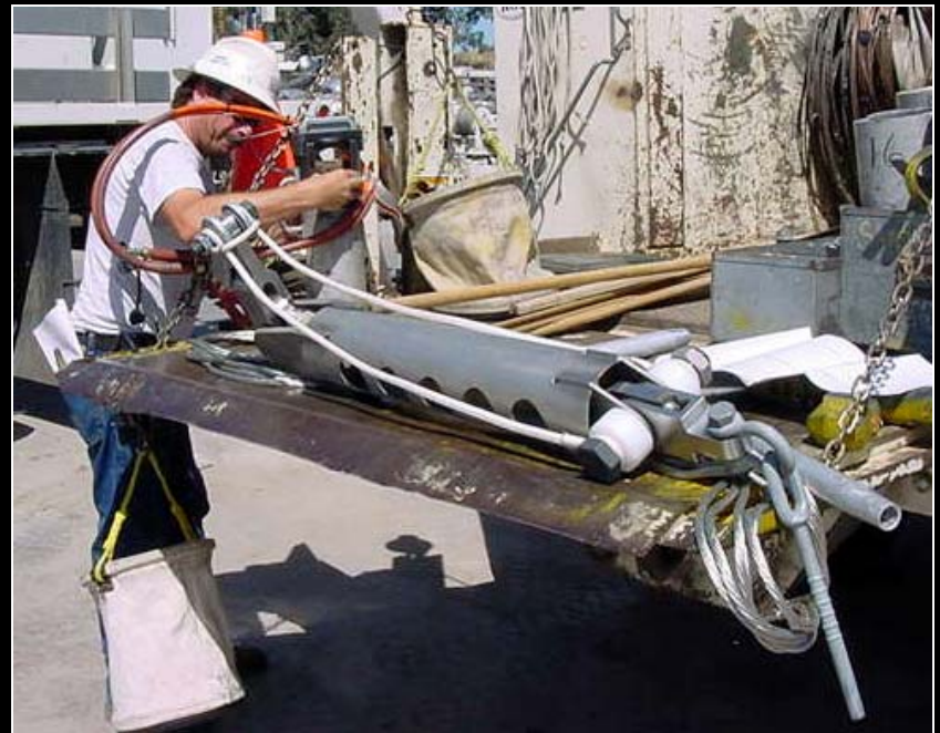
SLiM prepared for installation
