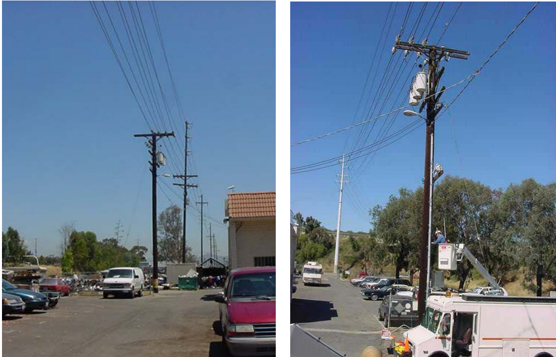
Figure 3: View of the test span, looking West (left photo) and looking East (right photo). Distribution pole is also evident.
