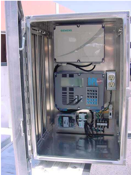
Figure 6: Controls for the Siemens monitoring
