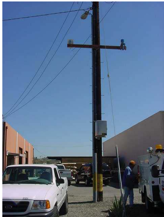
Figure 7: Monitoring equipment on the pole
